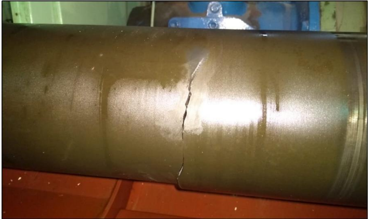
Picture #1 – Crack in the middle section of the coupling spool piece.
