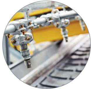
Fire extinguishing system
